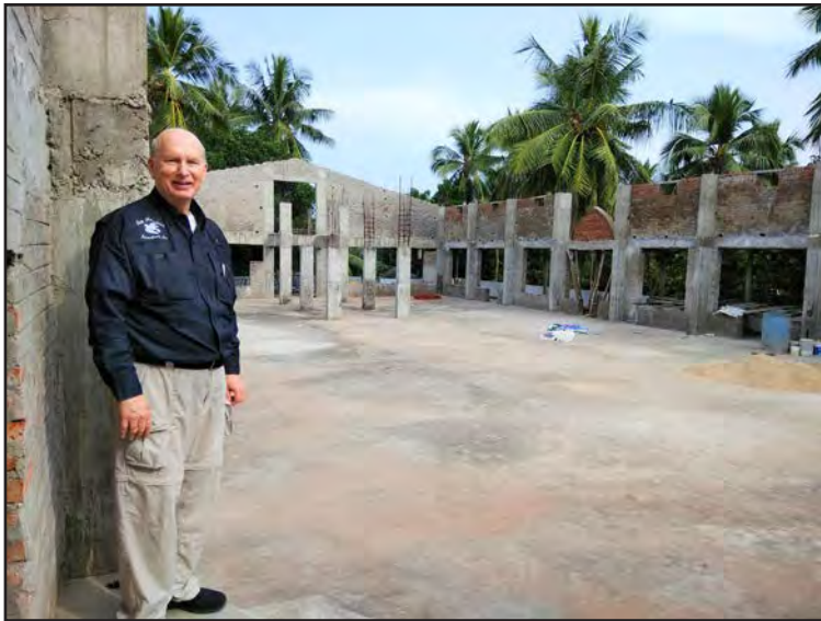
Standing at a church's new construction site after I preached a message on healing to a 1,000 plus people.
