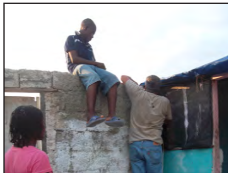
Tom & JoHannah worked on one of our Nanny's roof to keep the rain from pouring in!
