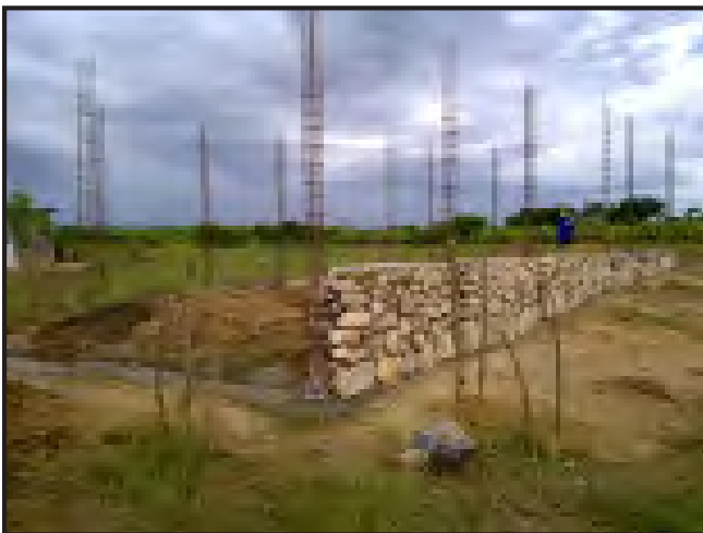
Work has begun on a permanent home for SCH!! This is an answer to prayer, and we are praising the Lord!
