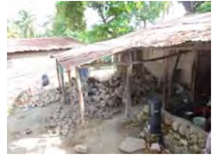
The back boundary wall that fell down during a recent heavy rain storm; building on left is next yard.
