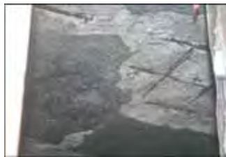
Patched ceiling with cement erosion
