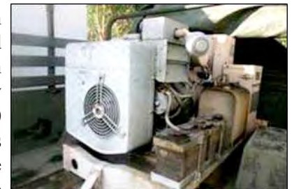
Our "new" diesel generator which will help many
